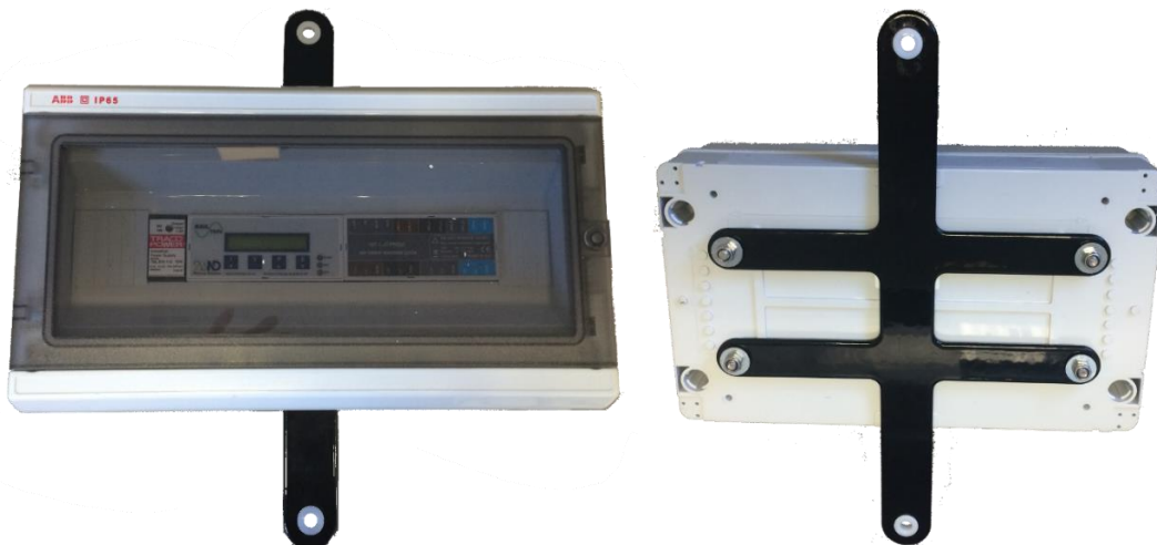
Figure 22 – Rail350v enclosure and double dagger bracket (for OHL pole mounting) front and rear view as used on the Lyndhurst EV trial cluster
