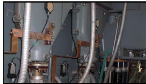
Figure 7 Switchgear equipped with sensors
