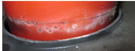
Figure 8 Bushings showing signs of discharges
