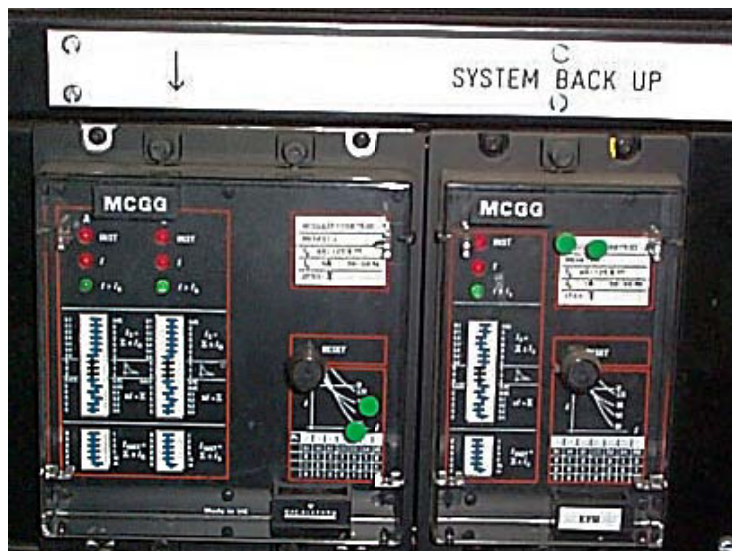
Figure 12 – View of New X 2 Back-Up Overcurrent & Earth Fault Relays at Wimbledon
