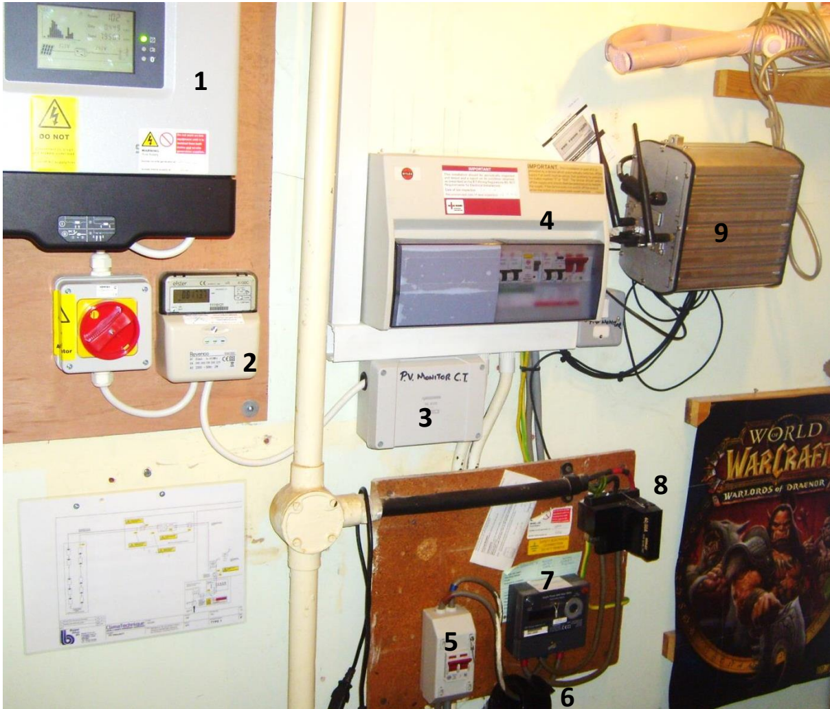
Figure 5 – Typical monitoring equipment setup
