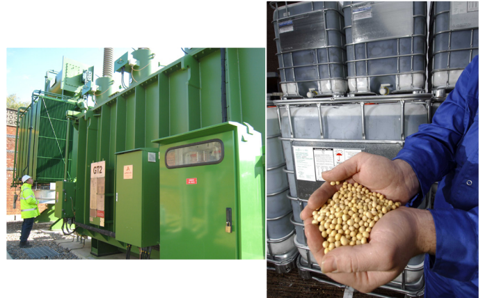
The green vegetable oil-filled transformer installed at a substation in north Luton. The fluid is made from edible seeds.
